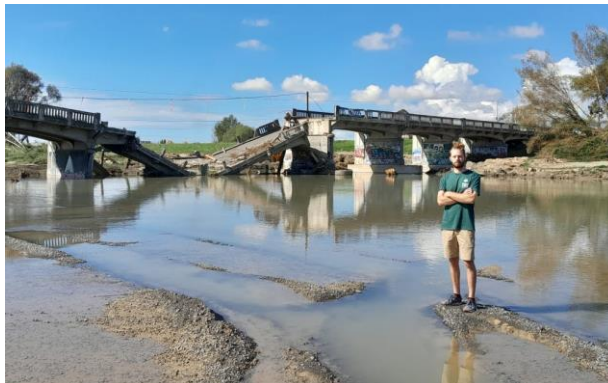
Redcliffe Bridge, Hawke's Bay, post Cyclone Gabrielle
